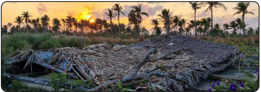
Church totally destroyed by Typhoon Ulysses
